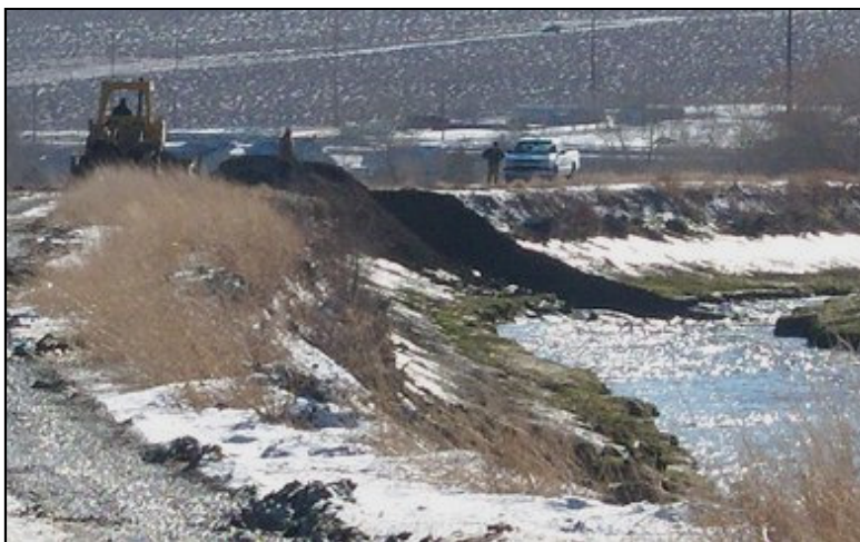
Last winter's levee break in the Truckee Canal that resulted in extensive flooding within the western Nevada community of Fernley has placed a spotlight on the nation's need to rehabilitate rapidly aging water infrastructure.
