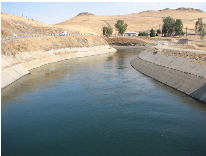
Friant Water Authority The Friant-Kern Canal, winding through the Sierra Nevada foothills northeast of Fresno.
